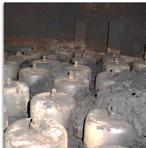
Figure 14 - Carbon Deposit Build up in a Gas Contactor 13
