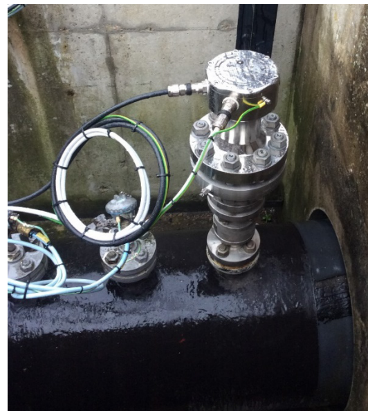
Figure 12 - Camera Can Mounted on a Gas Entry Point to the UK National Transmission System
