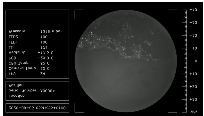
A view of the pipe below showing debris on the pipe floor
