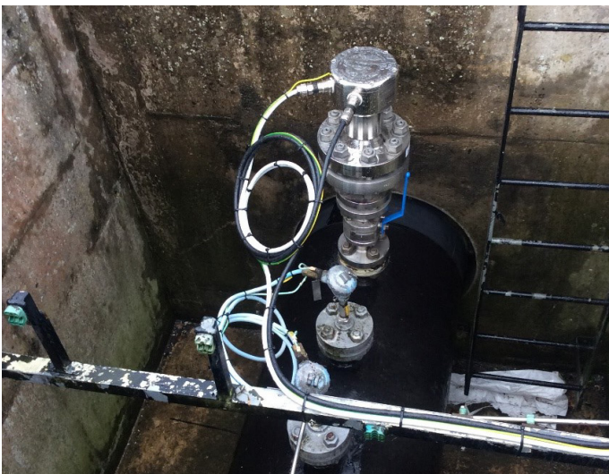
LineVu installation at an entry point to a gas network
